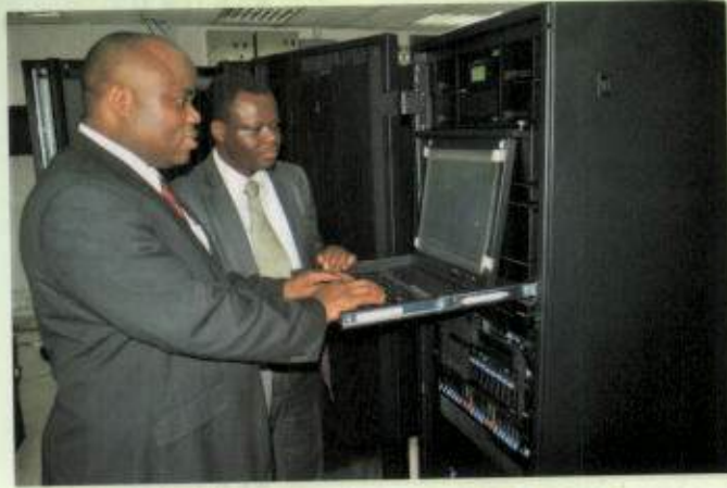
Server Room, CSCS Head Office
